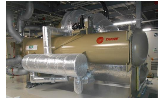
Centrifugal chiller with Non-Freon refrigerant
