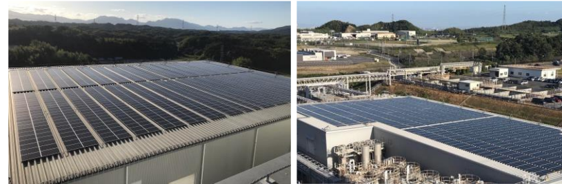
Solar power panel installed in Mie Plant
